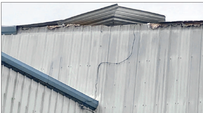
Roof damage from Nicole
